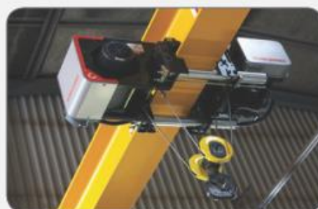
Example of a Powered Hoist
